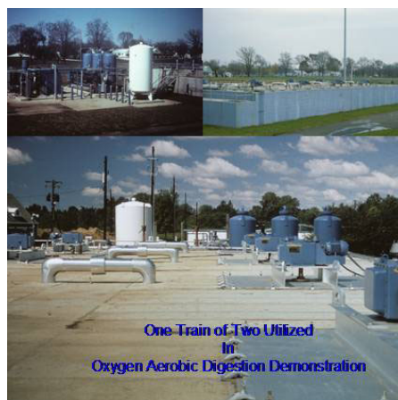
Figure 1 UNOX system at Speedway, Indiana
