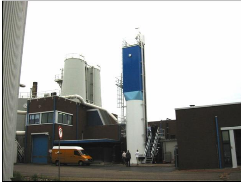
Figure 30 ANAMMOX Reactor at Rotterdam's Dorkhaven Plant
