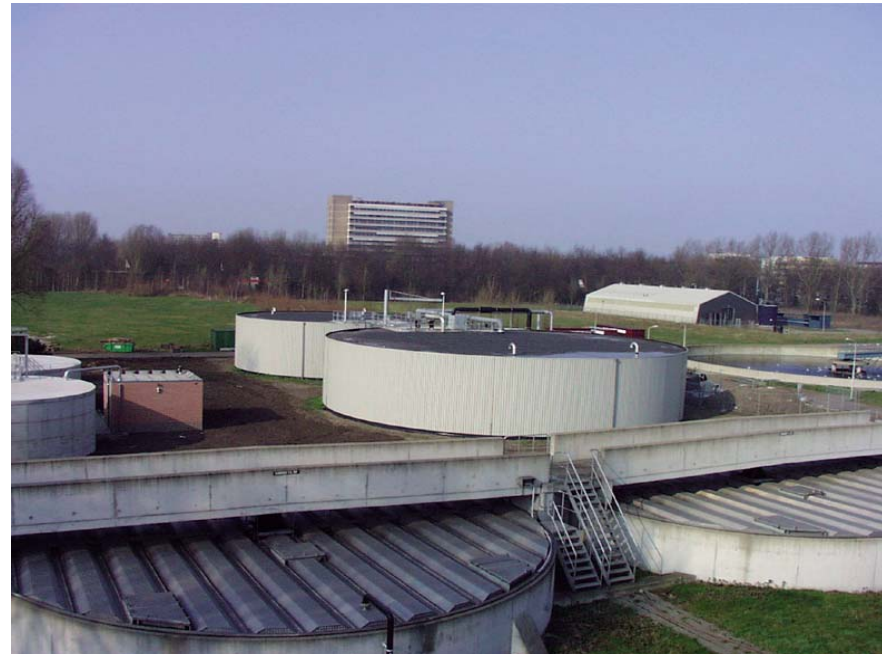
Figure 4 Nitrification reactor (foreground), denitrification reactor (background)
