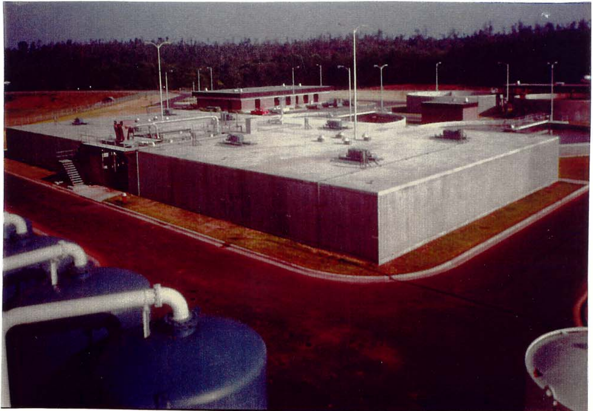
PSA Air Separator and UNOX R Nitrification Reactors
