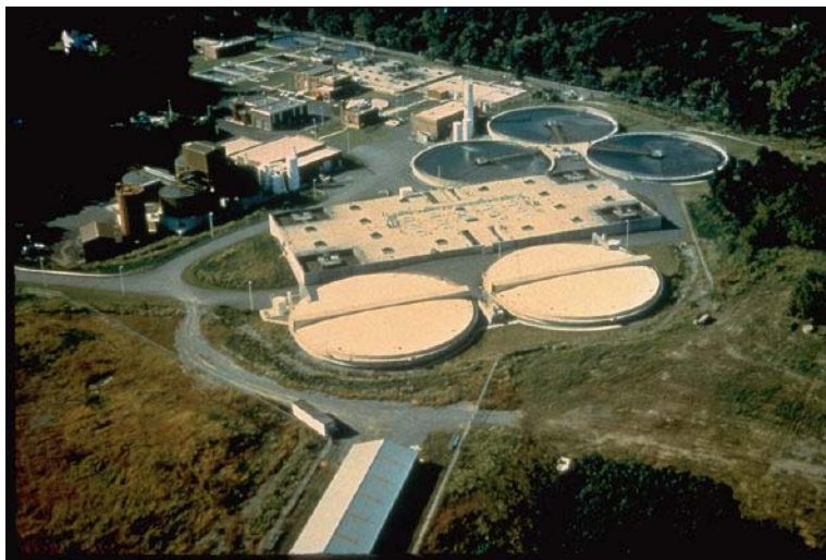
Lancaster, PA (North Plant in foreground)
