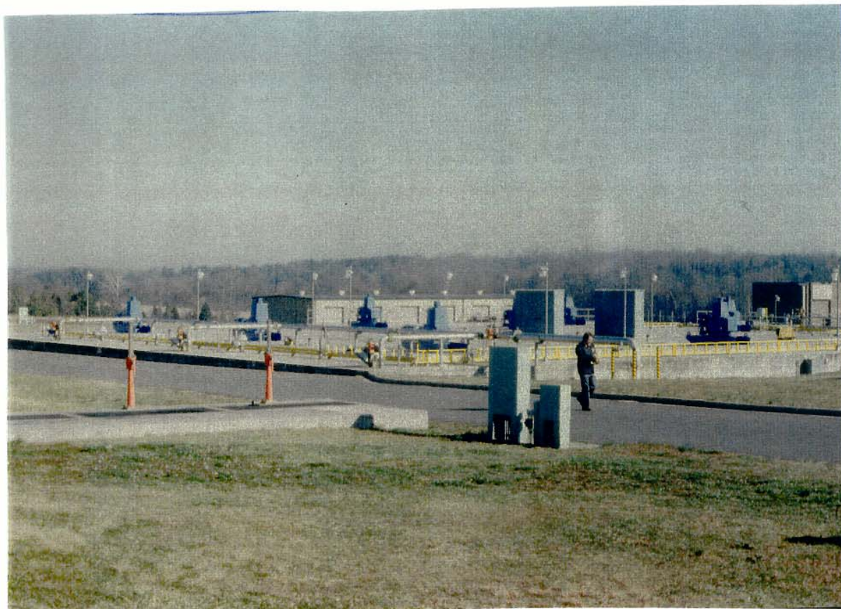
UNOX R nitrification reactors
