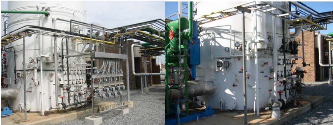
FIGURE 3 “U Plant” Controls After and Before Retrofit (Note installed I to P device rack)
