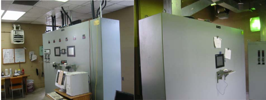
FIGURE 2 New Control Panels “U-Plant” (OPCP) and “UNOX” (HBCP)
