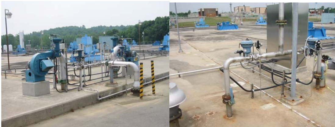
FIGURE 1 Converted Oxygen Feed and Vent Control Subsystems (note use of globe feed and ball vent valves)
